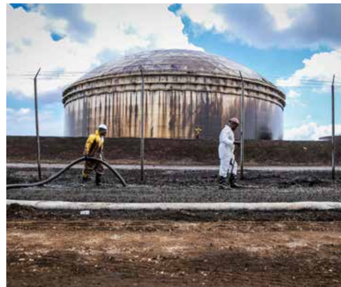
HIT HARD: In 2019 the Bahamas was turned upside down by Hurricane Dorian, the worst natural disaster in the archipelago's history. 74 people lost their lives, and the storm led to major damages to infrastructure, people, and the local environment. Photo: Zak Bennett / AFP.
