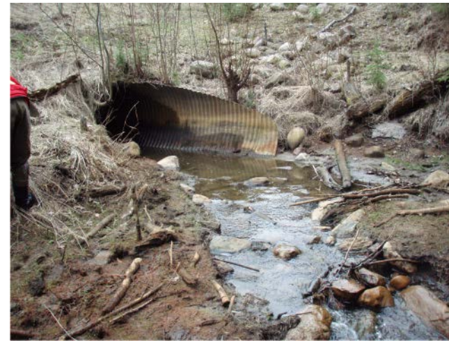
PHOTO 1. Culvert and road crossing at the upstream section of the study reach (May 2007)
