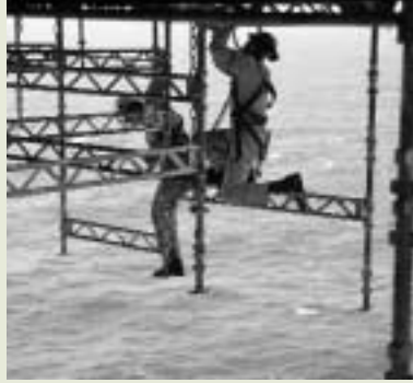
Forty installations, on land and offshore, have gone through Statoil's most rigorous safety testing ever. This led to methods for monitoring the condition of the facilities throughout their lifetime, which will help the operations organisations to maintain a high standard.
