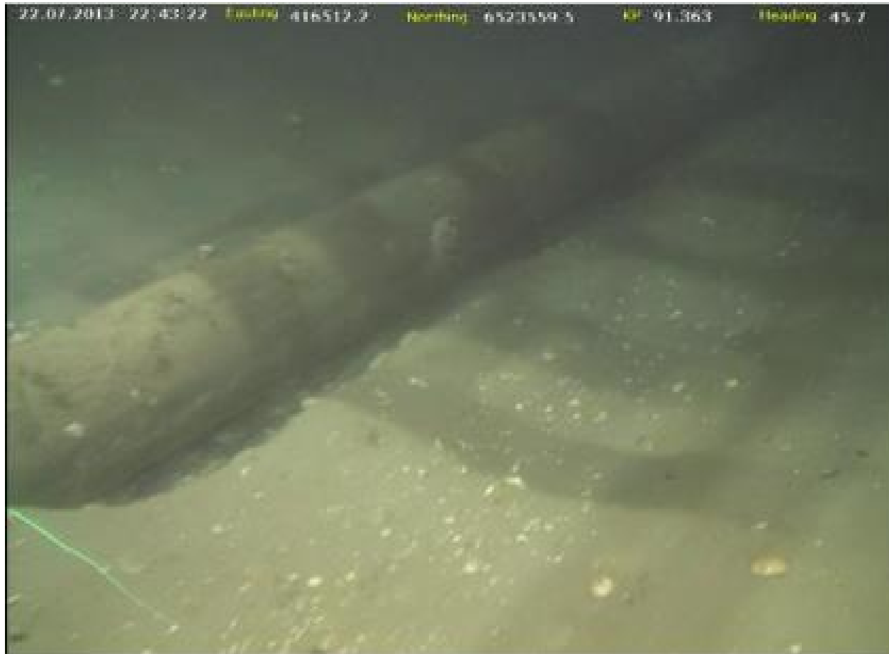
Figure C-3 Image from 2013 pipeline survey at KP 91.363 showing section of PL301 exposure within the trench
