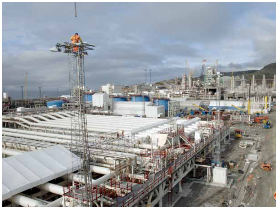
Statoil is building Europe's first plant for the export of liquefied natural gas (LNG) on Melkøya off Hammerfest.
