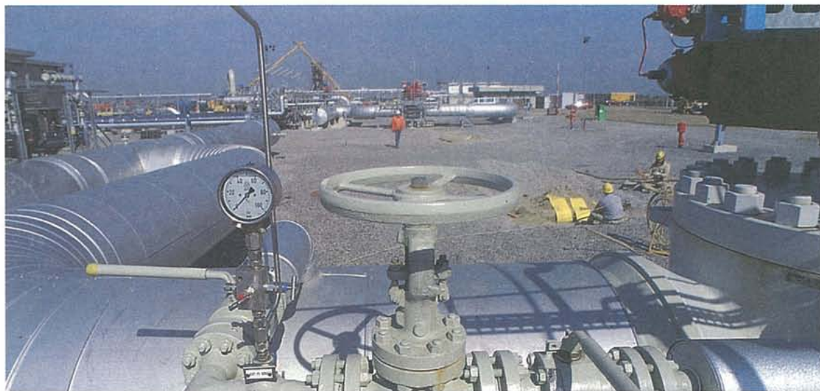
Metering gas from the Norwegian continental shelf as it reaches Germany through Europipe.
