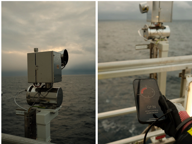
Figure 9: The CCTV camera mounted on turbine HY06. Pictures taken by an Equinor operations engineer 7 March 2024.
